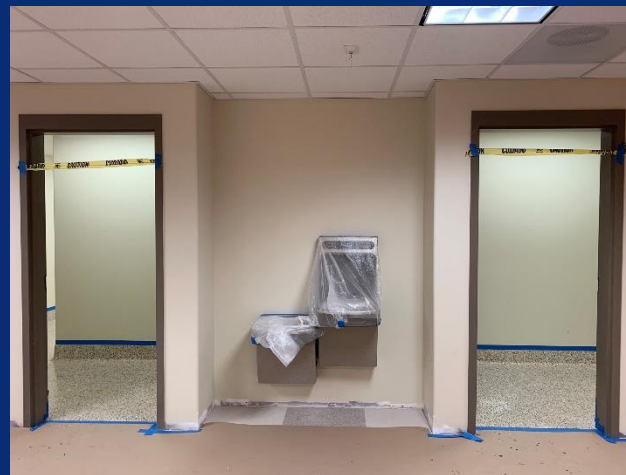
Drinking Fountain in Area F
