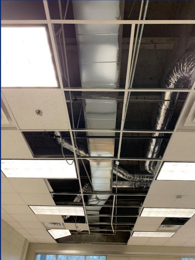
Exhaust Vent in Area G
