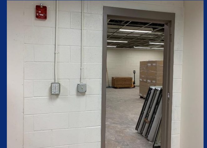
Wall Devices in Area K
